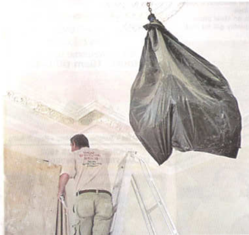
► PAINSTAKING WORK BEECHWORTH BED AND BREAKFAST FREEMAN ON FORD HAS UNDERGONE EXTENSIVE RENOVATIONS.
